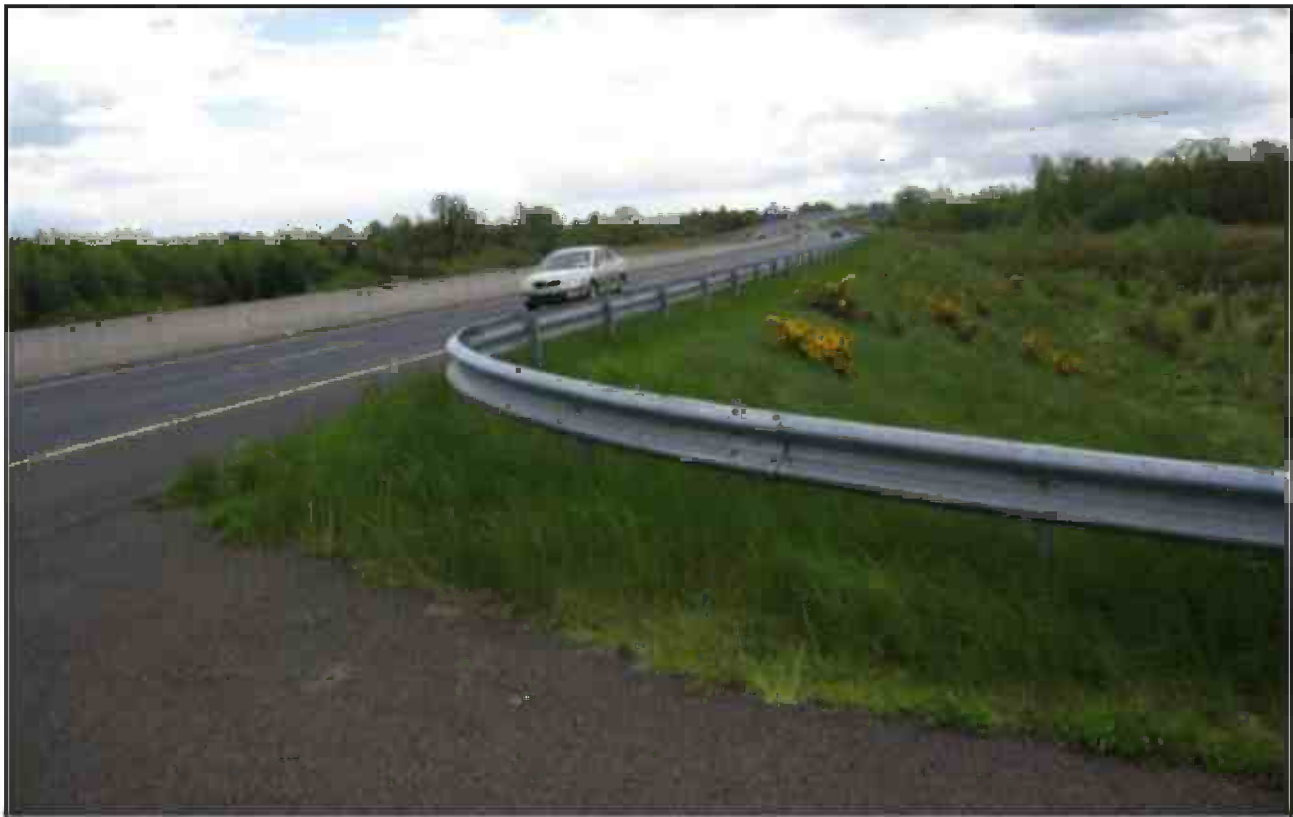
Entrance to attenuation pond from M7 eastbound carriageway.
