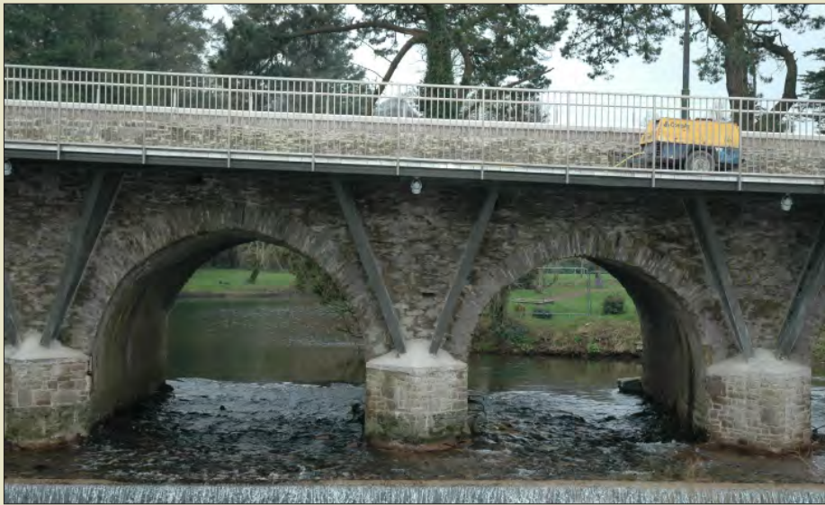
Looking south at detail of partly rebuilt cutwaters with struts supporting footbridge decking. (Photo: Ken Hanley)
