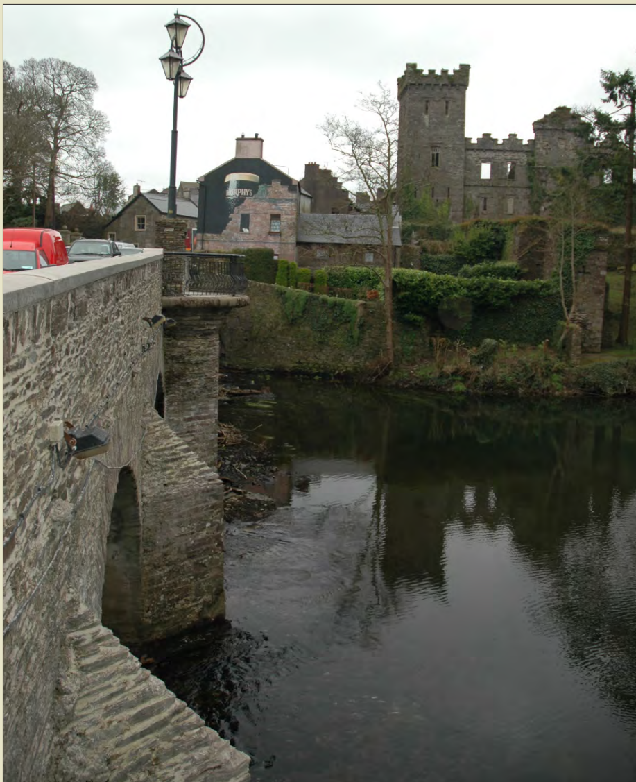
Southern side of bridge following cleaning and re-pointing, with site of Macroom Castle in the background. (Photo: Ken Hanley)
