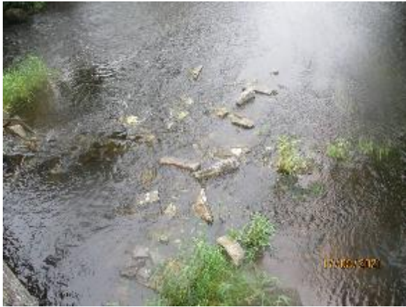
Plate 3. Castlereagh Bridge. Instream debris resulting from fallen masonry parapet wall.
