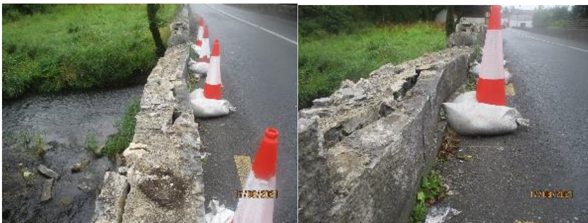
Plate 2. Castlereagh Bridge. Damaged parapet wall and fallen debris highlighted in red.
