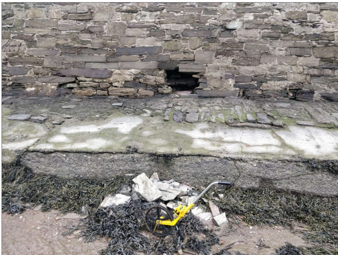
Plate 3-4 – smaller section of retaining wall to be repaired.
