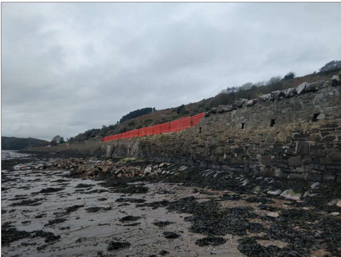
Plate 3-1 – View of the collapsed parapet looking northwest.
