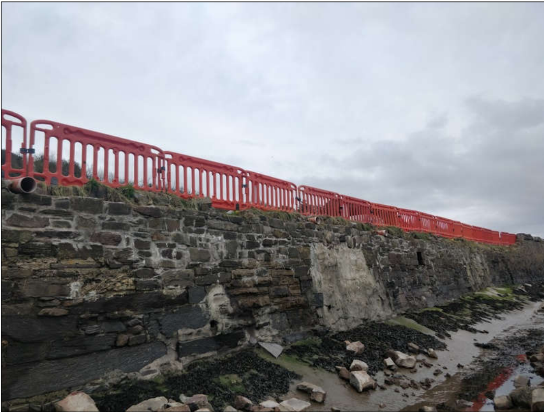
Plate 3-2 - Close up of collapsed parapet.
