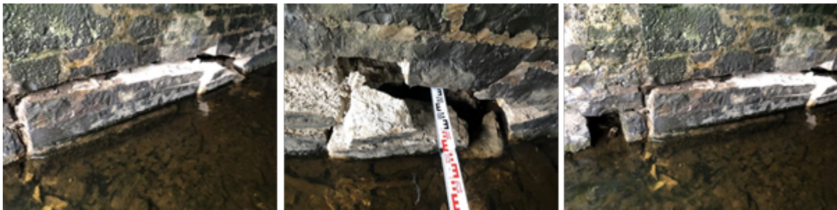
Plate 1.2 Damaged abutment at River Suir Bridge.
