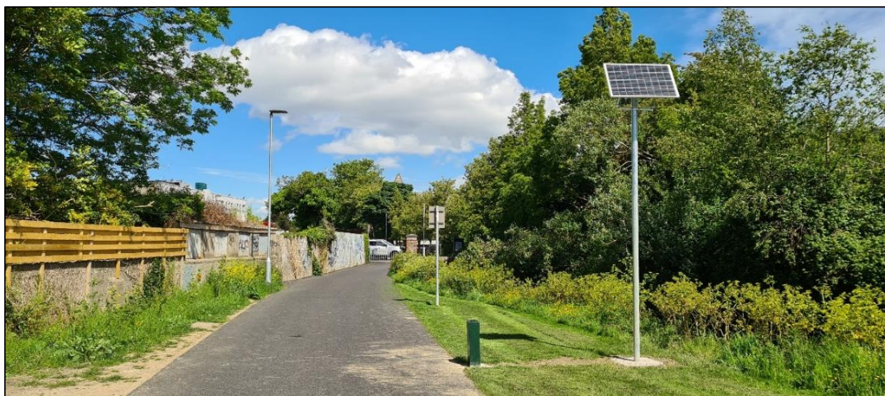
Figure 8.1 Example of the supporting infrastructure for an automatic counter
