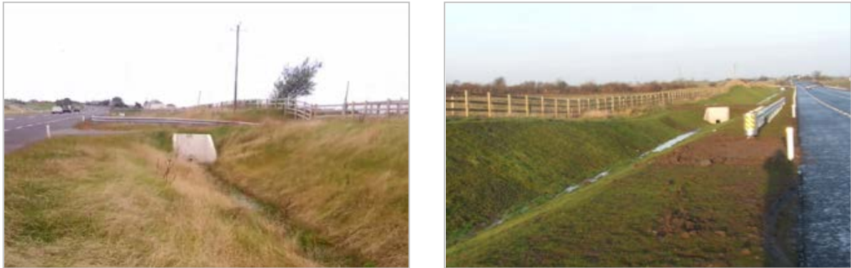
Figure 8 - Examples of hazardous drainage features
