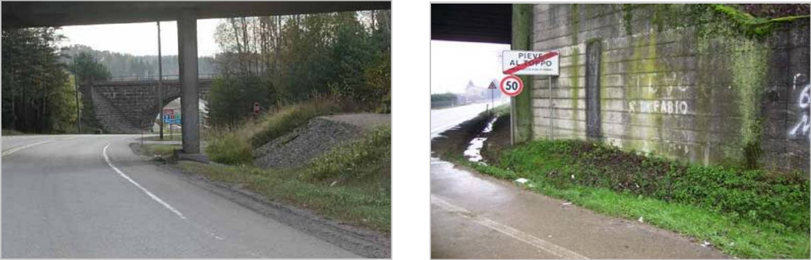
Figure 5 - Examples of a hazardous bridge abutment (left) & overpass (right)
