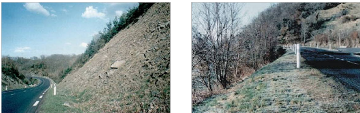
Figure 9 - Examples of hazardous cut (left) and fill slopes (right)
