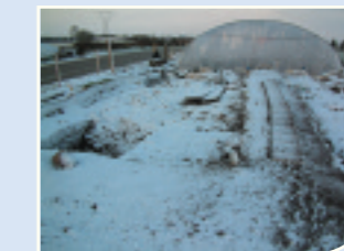
Excavating at the Ballykilmore enclosure during winter. (Photo Valerie J Keeley Ltd)
