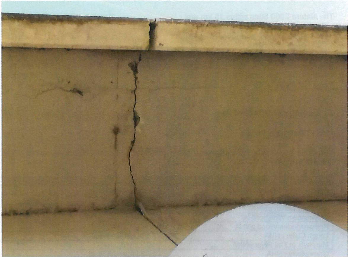
Plate 2. Damage to girder
