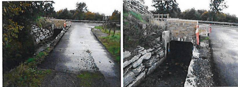
Plate 1. Upstream of Killygordon Culvert with damage parapet to right.
