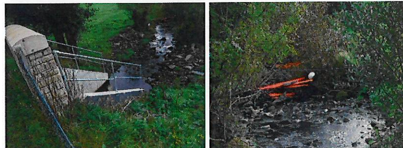
Plate 3. Downstream headwall & debris in river downstream of culvert. [Source: Atkins R.E.; 1/10/2018]
