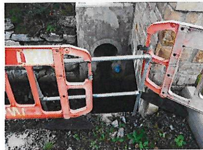
Plate 2. Outfall at upstream side of culvert; safety fence along damaged parapet.
