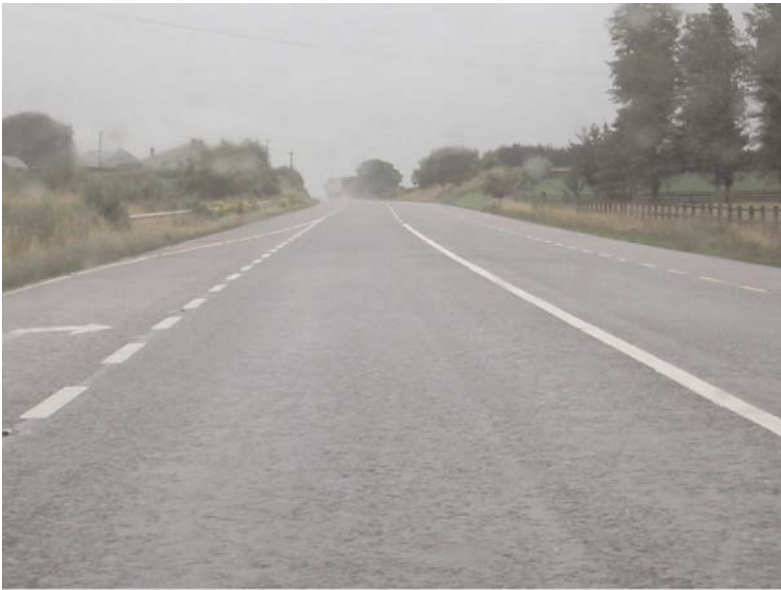
Before road safety remedial measure implemented
