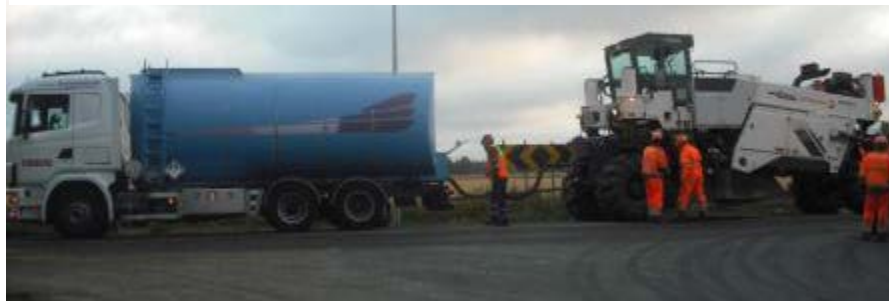
Bitumen tank in front of the WR recycler
