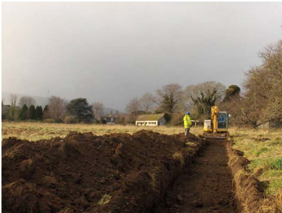
Plate 2: Trench 11 during excavation. Looking west towards Priorsdown House, stables and an approaching heavy rain shower.
