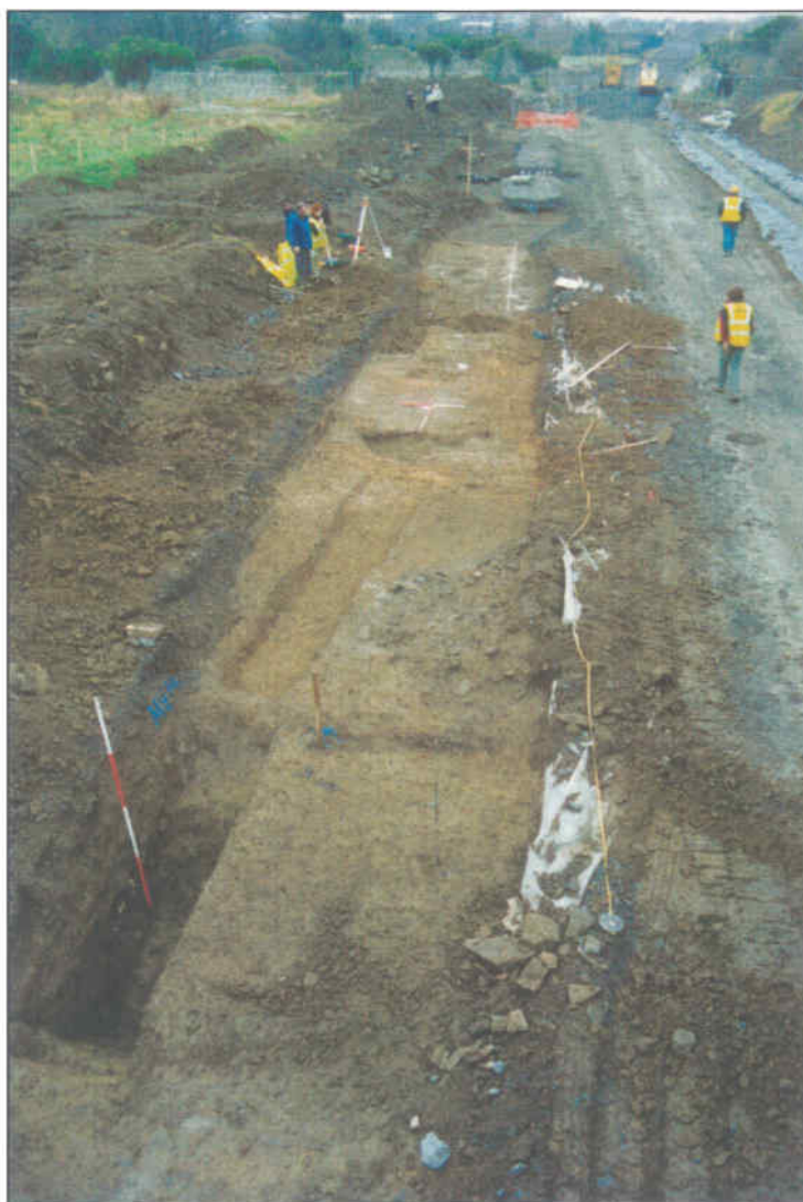
Plate 3 Strip of ground at southern end of site excavated in January 2002. Phase II field drain (F32) to lower left side and metalled surface (F23) to centre
