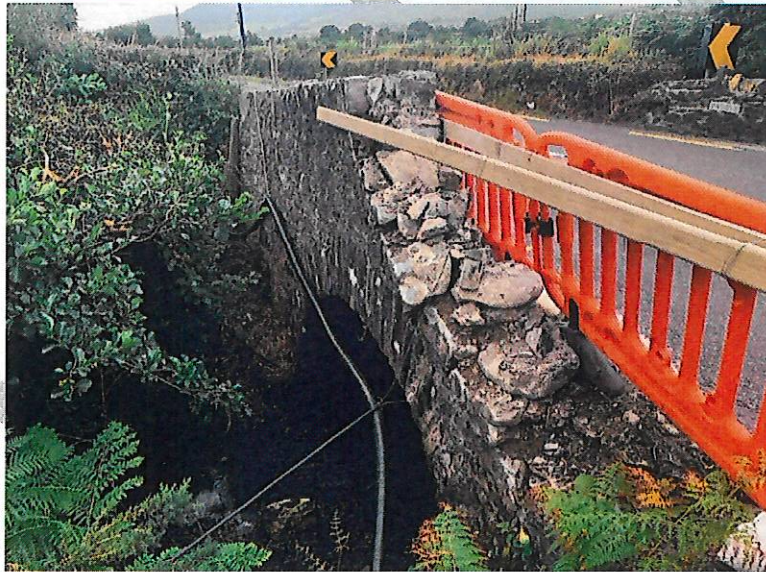
Plate 1. Damage to parapet wall on northern side of the N70.
