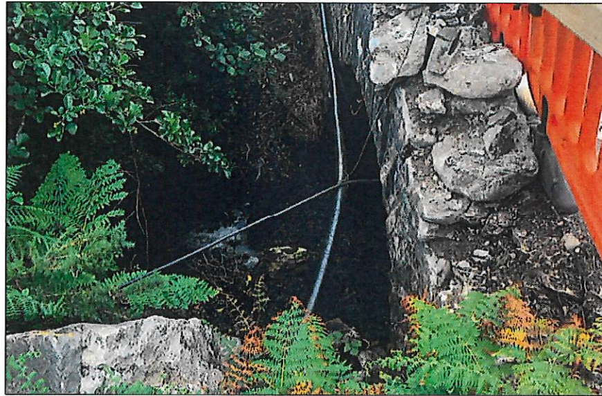
Plate 2. Damage to parapet wall on northern side of the N70.
