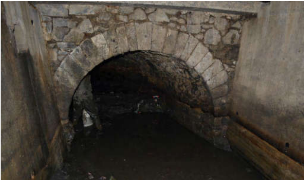
Plate 4.6 View through the culvert looking at West Elevation of Masonry Section (from RPS, 2017).
