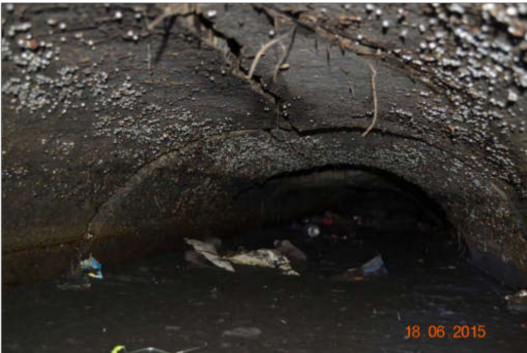
Plate 4.10 View through outfall pipe. Failed pipe units to be replaced (from RPS, 2017).
