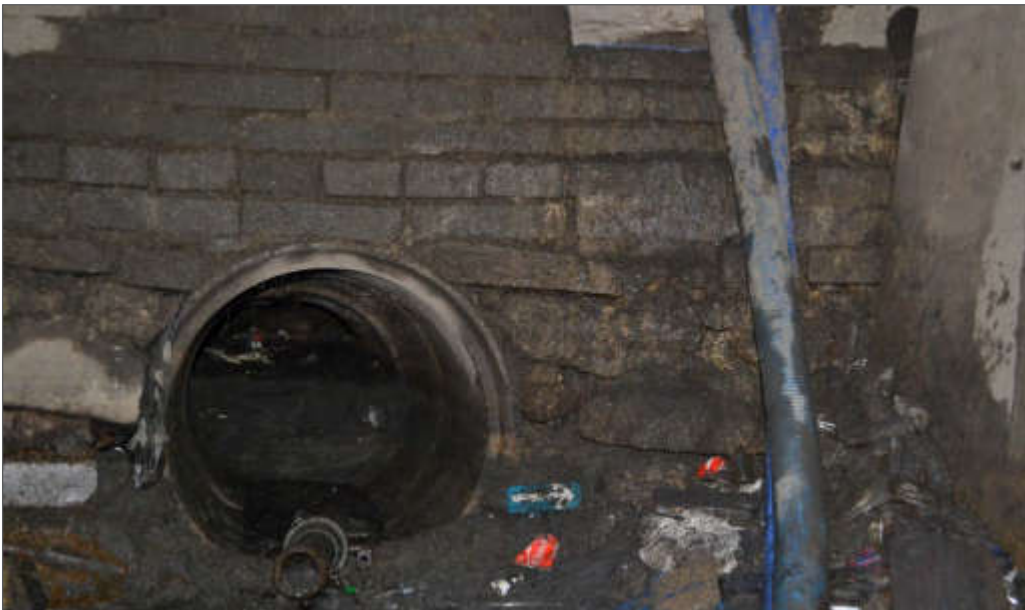
Plate 4.8 West face of box culvert at interface with outfall pipe (from RPS, 2017).
