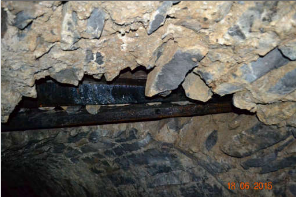
Plate 4.11 Ductile iron watermain crossing through the crown of the arch barrel (from RPS, 2017).
