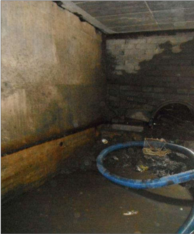
Plate 4.7 West face of box culvert at interface with outfall pipe (from RPS, 2017).
