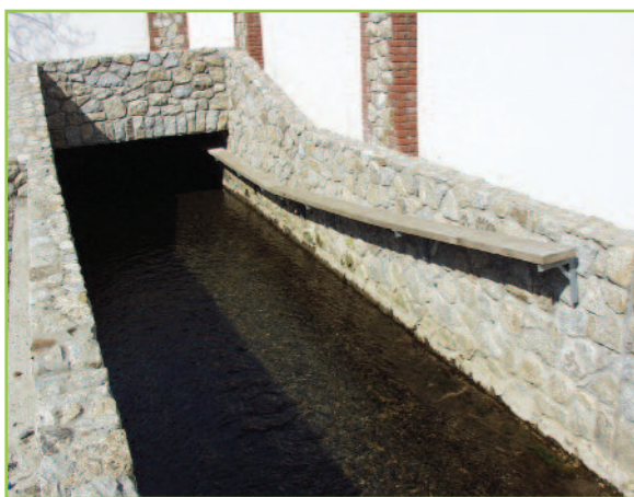
A culvert with an otter ledge attached on brackets. This section of artificial channel has a stonepitched base on which sand and gravel will lodge more readily than concrete.
