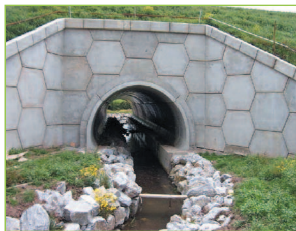
An example of a well designed oversized arched culvert with mammal ledges. The natural bed of this watercourse was maintained.
