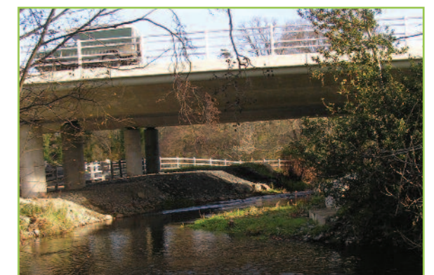
A well designed clear-span bridge retaining the existing river channel with piers set back from the river bank.
