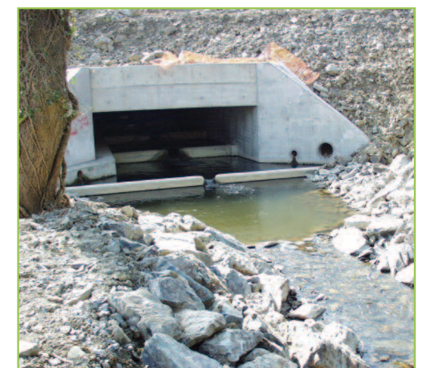
A well designed culvert which has a stepped profile to accommodate fish passage and an outlet pool to allow fish to pass upstream into the first of the steps. The culvert incorporates a cast mammal ledge.
