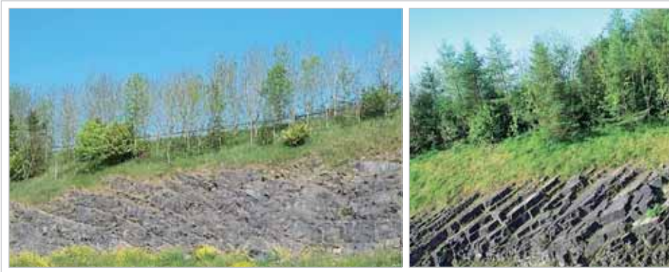
Figure 2-1: N4 Mullingar Bypass. The road cutting along the N4 Mullingar Bypass exposed a superb anticline fold in the Carboniferous limestones. As traffic enters the cutting, limestone beds dip one way and then level out at the top of the cut before dipping away in the opposite direction. This excellent visible demonstration of simple geological phenomena such as beds and folds was for a period rendered invisible by roadside planting.
