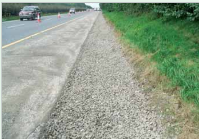
Figure 5-9: Example of a French Drain on M4
