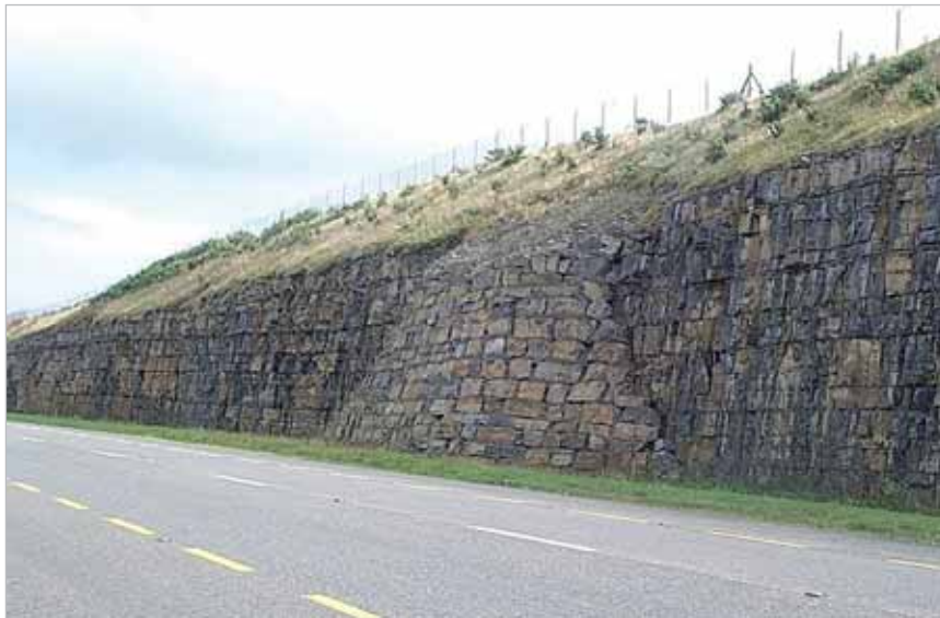
Figure 1-2: N17 Claremorris By-pass. A localised depression in the bedrock (infilled dissolution feature) was encountered in a steep sided rock cutting developed in horizontally bedded limestone along the N17 Claremorris Bypass. The soil encountered in the steepened side slope was retained behind a wall faced with limestone blocks in order to achieve a uniform geological profile within the rock cutting.
