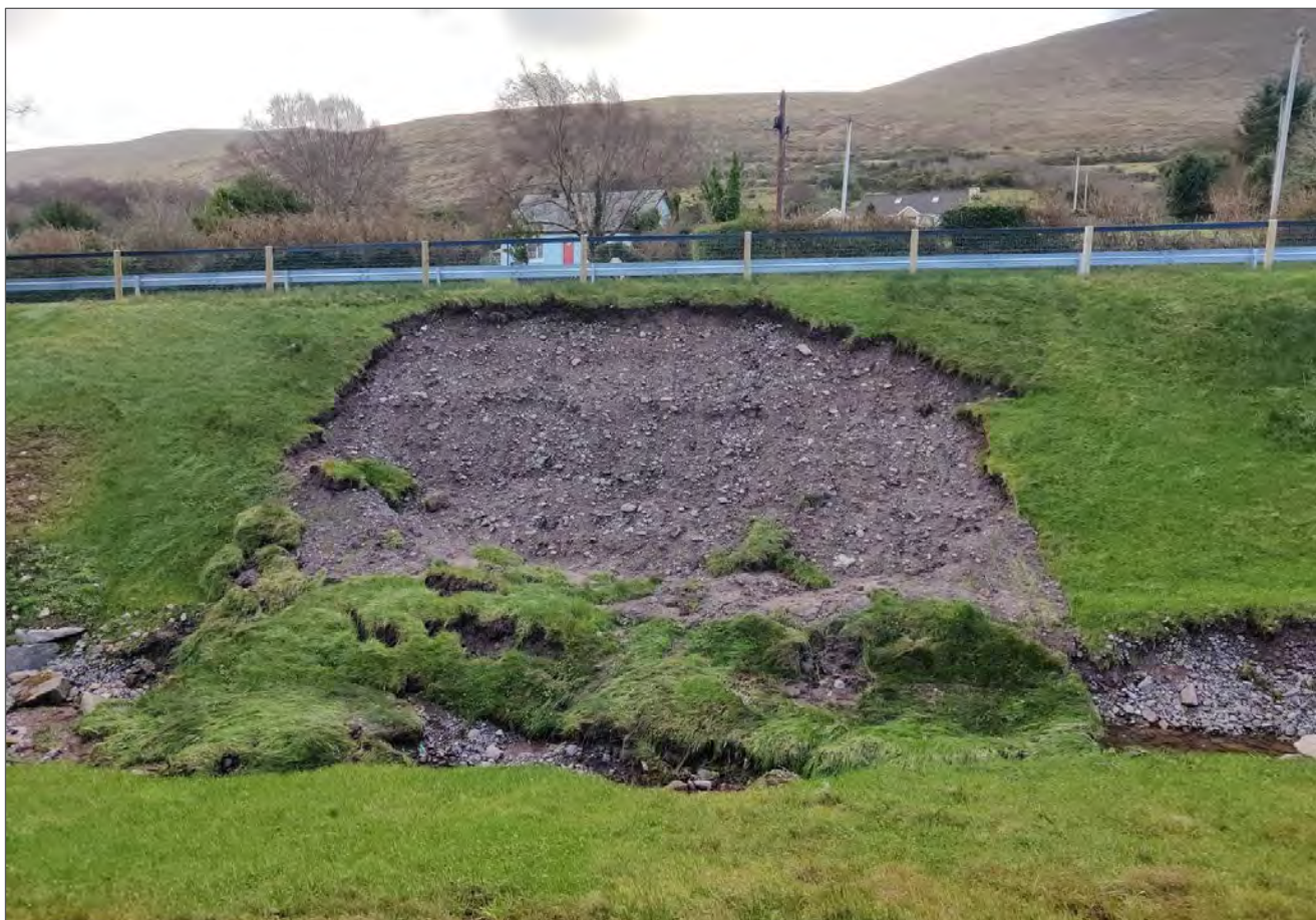
Figure 1-3 - Topsoil slippage in January 2024.
