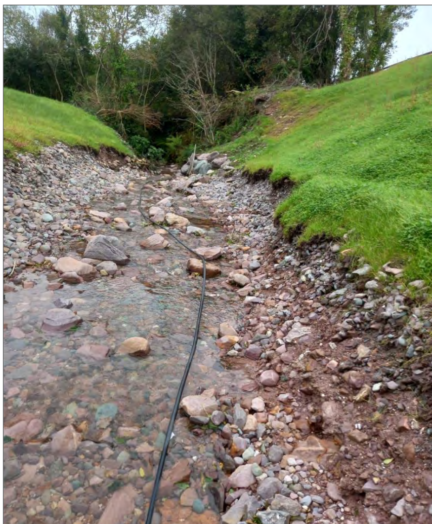
Figure 1-2 - Erosion and scour in the stream channel and embankment toes in October 2023 (prior to topsoil slippage from the right-hand side in this photograph).
