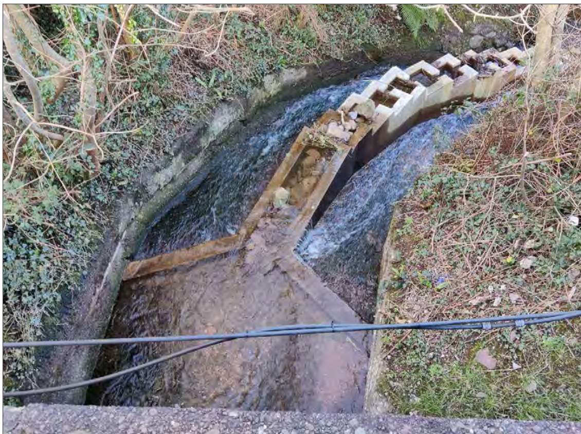
Figure 1-5 - New fish pass blocked by stones and debris.
