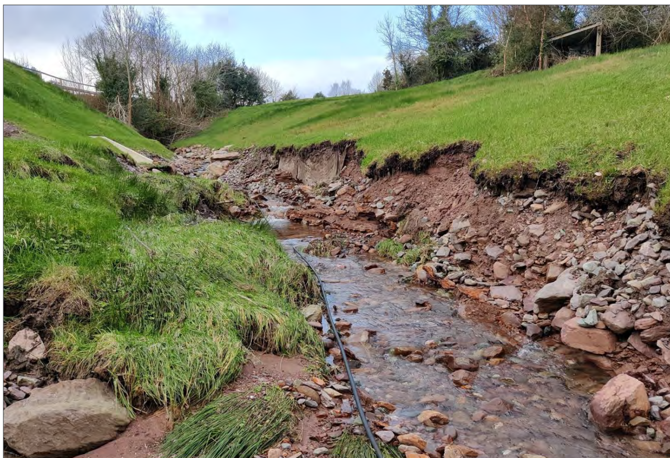
Figure 1-4 - Erosion of the toe of the opposite embankment due to deflection of the stream by slumped topsoil from the roadside embankment.
