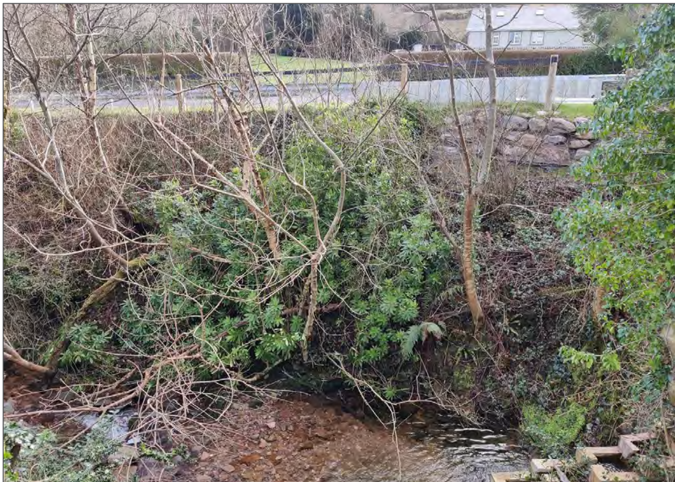
Figure 4-5 - Remaining Rhododendron on the roadside embankment just downstream of Curraheen Little Bridge, outside of the works area (January 2024).
