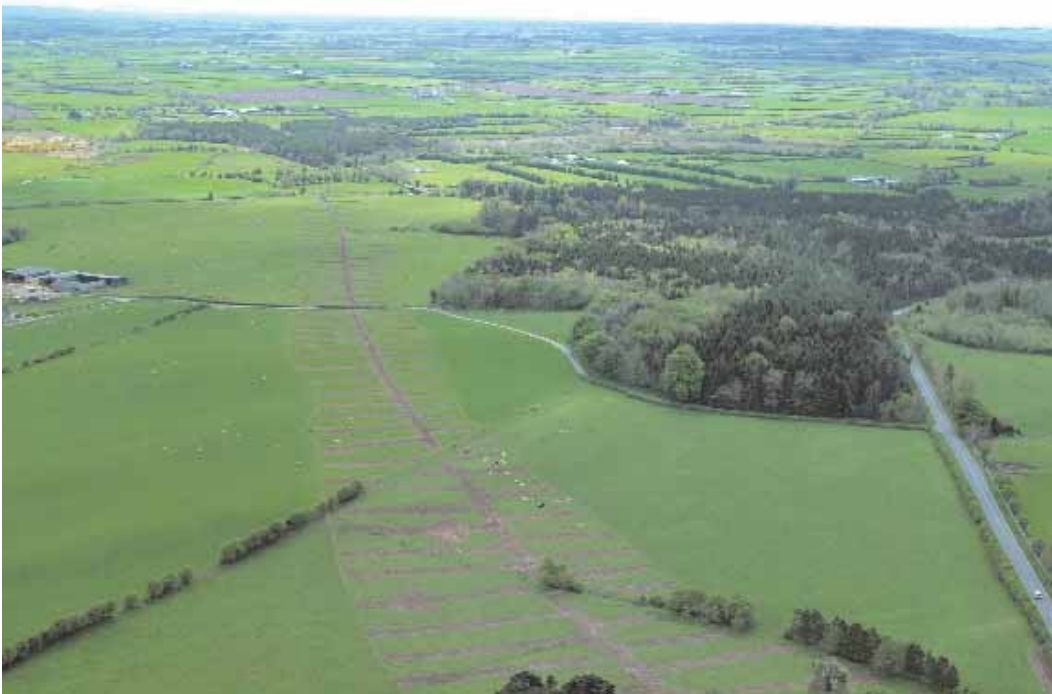
Illus. 3—Centreline testing on a section of the M7 Portlaoise–Castletown/M8 Portlaoise–Cullahill motorway scheme (Narrowcast)
