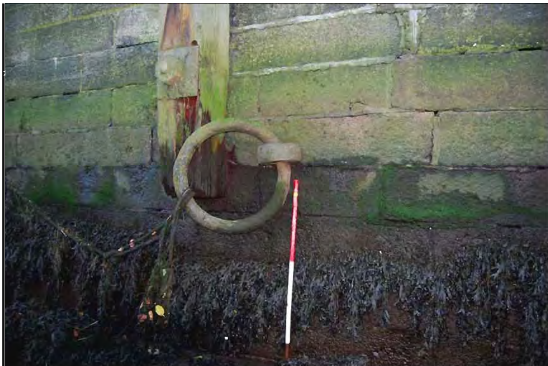
Plate 19: Detail shot of nineteenth century iron mooring hoop located along the HWM of Burgh Quay (1m scale).
