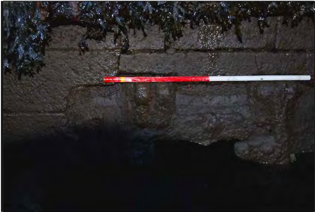
Plate 20: Detail shot of top section of nineteenth-century drain located along the base of Burgh Quay (1m scale).
