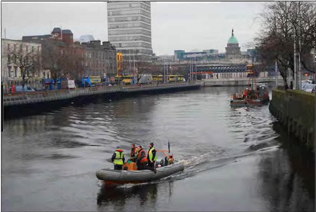
Plate 1: East-facing view of downstream side of O'Connell Bridge; dive boat in foreground and drilling platform in background.
