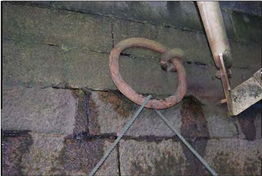
Plate 30: Detail shot of iron mooring hoop located along HWM of Eden Quay (Feature 3).
