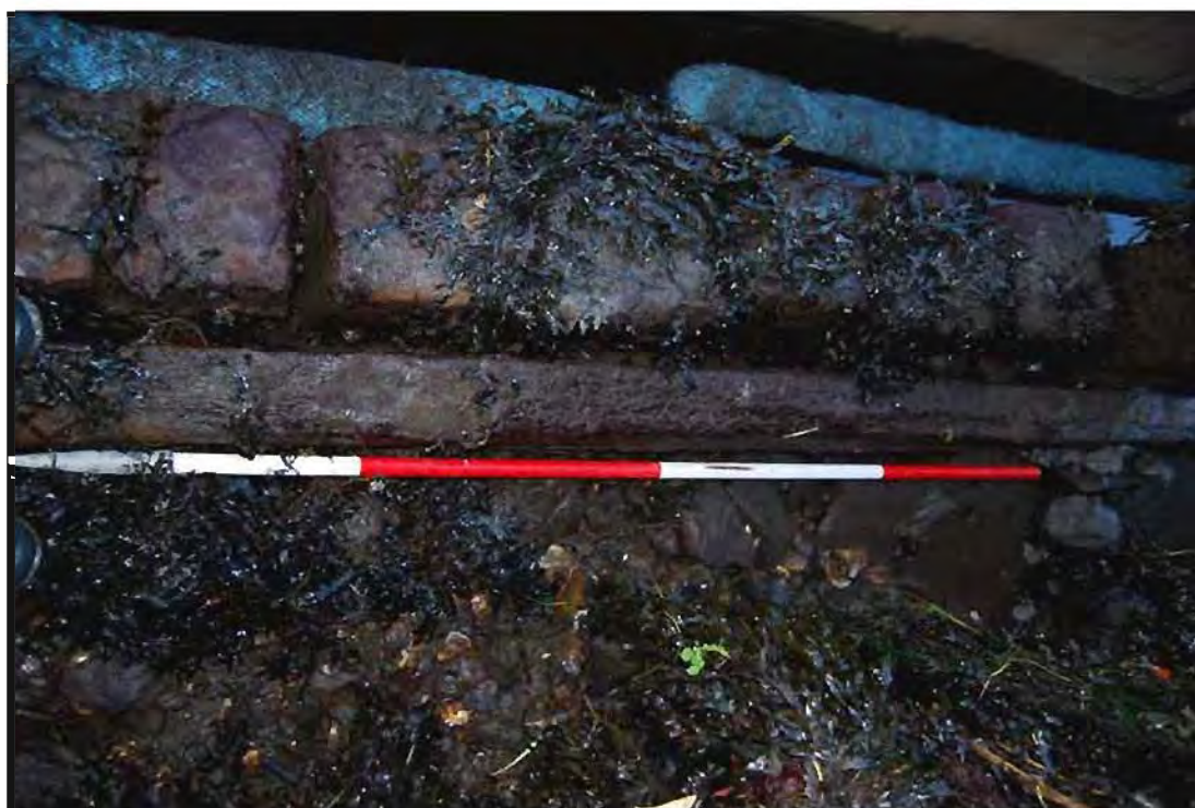
Plate 28: Plan view of timber vertical timber piles (Type A) and adjacent horizontal timbers (Type F); 2m scale.
