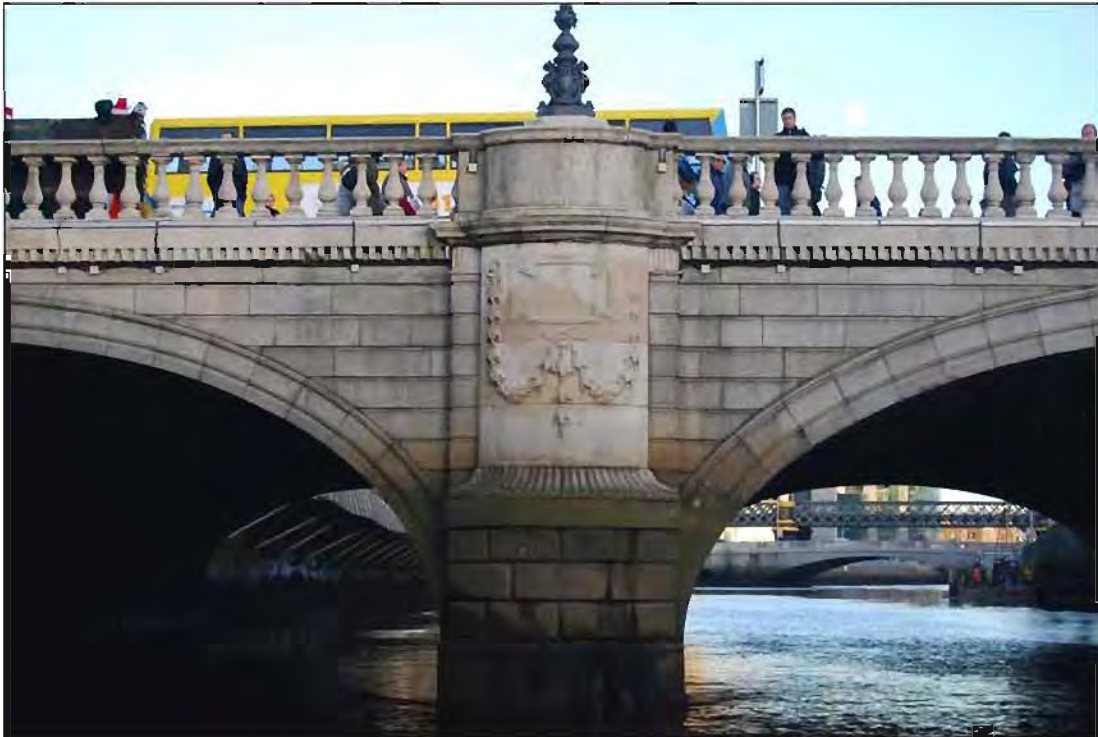
Plate 3: East-facing view of upstream cutwater, located between the northern and central archway.
