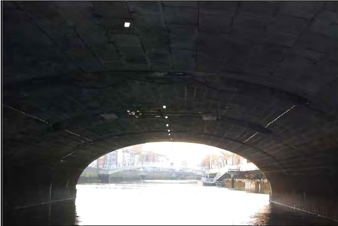
Plate 5: West-facing view of arch intrados (internal-arch ceiling) of the central-arch of O'Connell Bridge.
