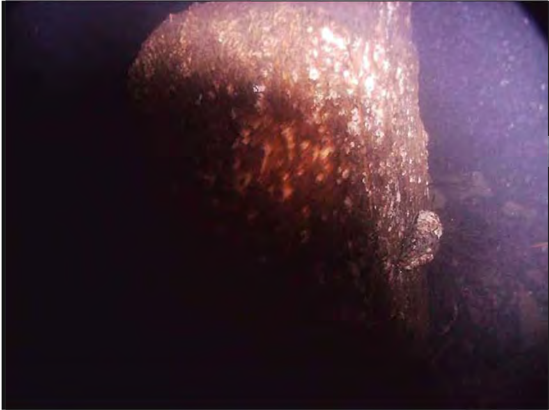
Plate 14: West-facing view of top of timber pile upstanding 0.60m from riverbed, c. 0.85m from arch-wall on north side of central archway.
