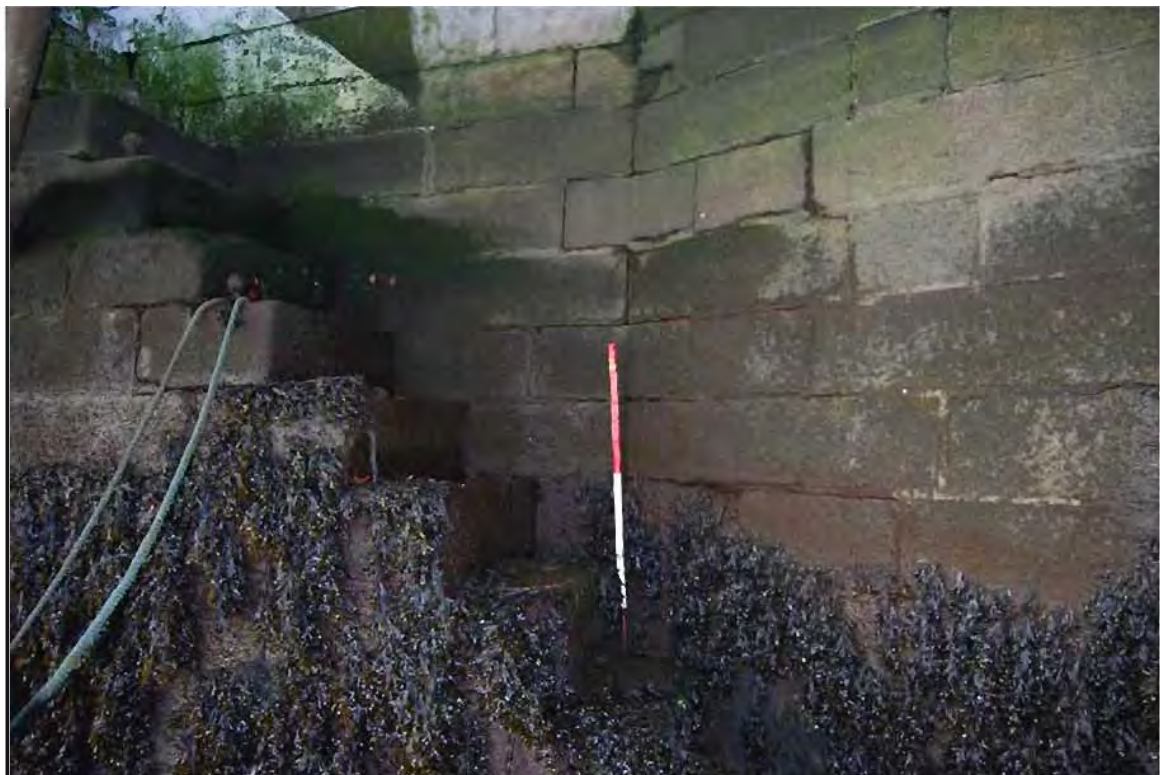
Plate 33: North-facing view of masonry steps providing access to the river from Eden Quay (Feature 3); 1m scale.
