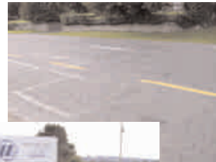
Example loops embedded under road pavement
