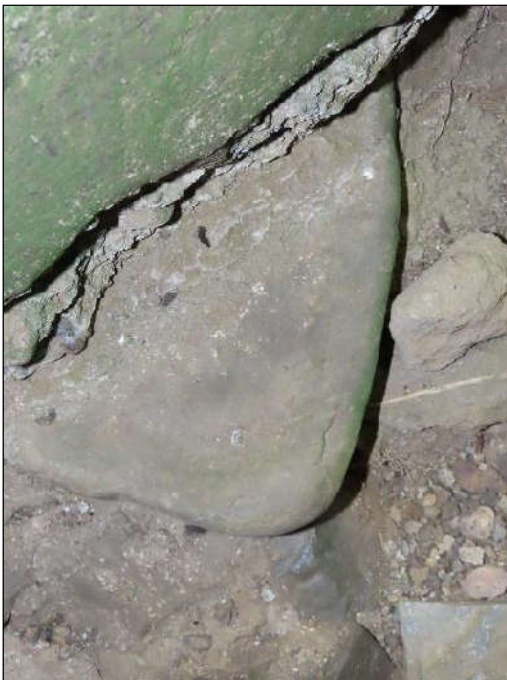
Plate 4.3 Small number of bat droppings on floor of easternmost span.
