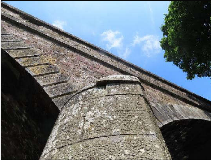
Plate 4.14 Stonework of downstream pier between easternmost and centre arch, no open crevices for bats.
