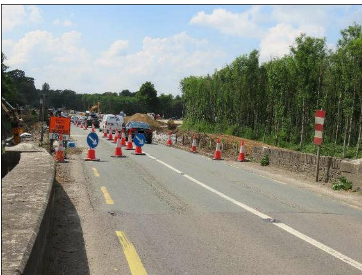
Plate 4.34 View looking west showing proximity of road widening works to Leader's Bridge and especially the Western Flood Pass.
