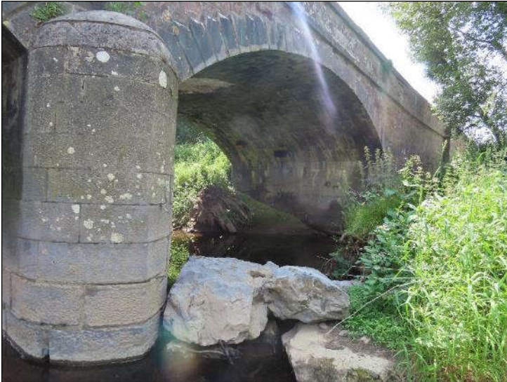
Plate 4.17 Westernmost arch – large rocks at upstream side of arch.
