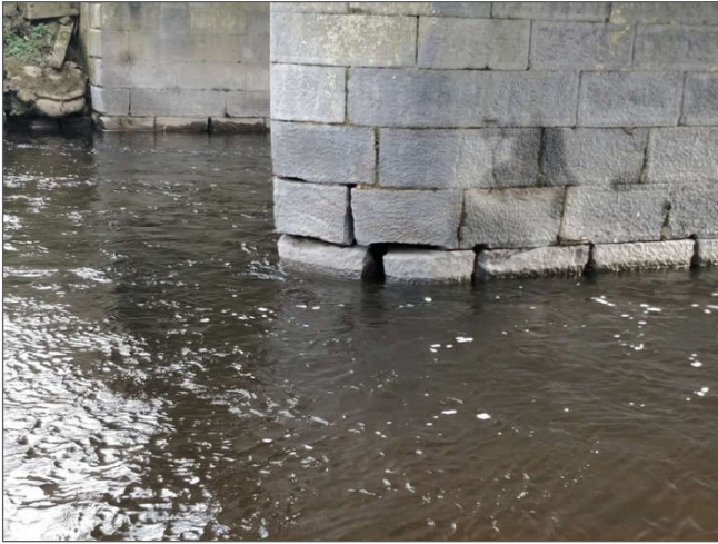
Plate 1.7 Masonry damage of north cutwater of east pier.
