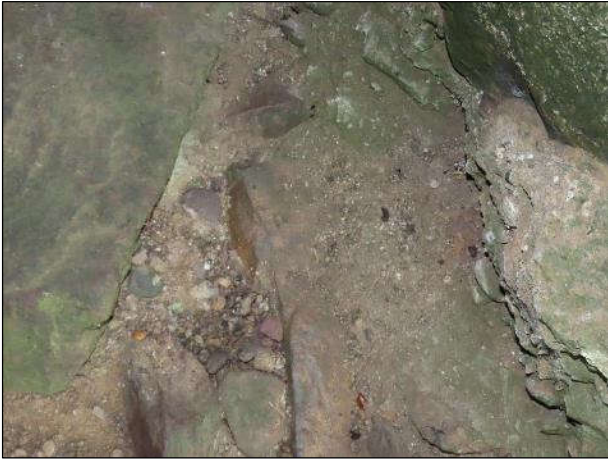
Plate 4.2 Small number of bat droppings on floor of easternmost span.
