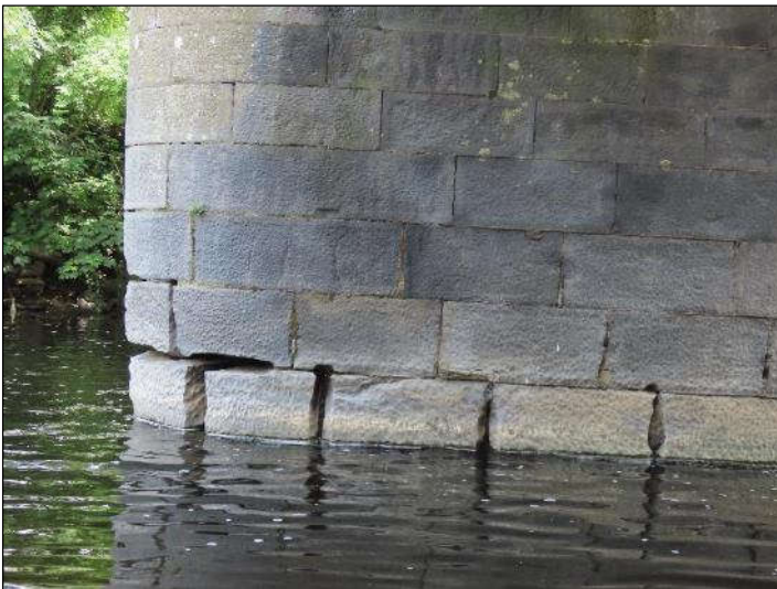
Plate 4.16 Close-up of movement of stones at base of abutment and pier of centre arch.
