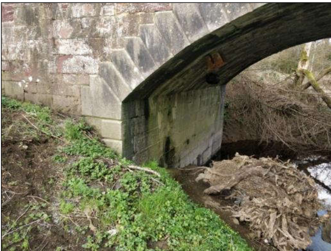
Plate 1.2 Blocked western span of Leader's Bridge.
