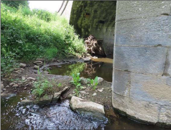
Plate 4.23 Mud bank at downstream face of western arch.
