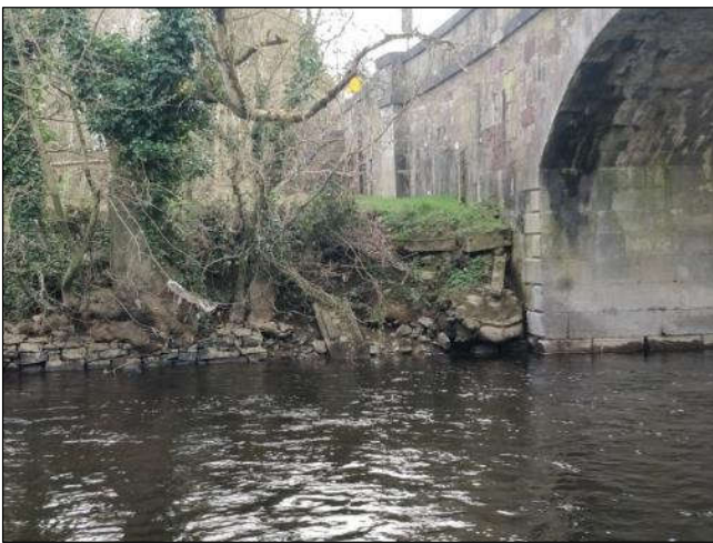
Plate 1.8 View of damage on embankments.
