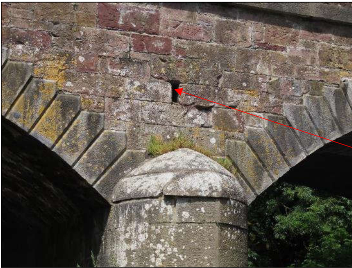
Plate 4.15 Void above downstream pier. A grey wagtail was recorded flying out from this void in the downstream (southern) bridge wall.
