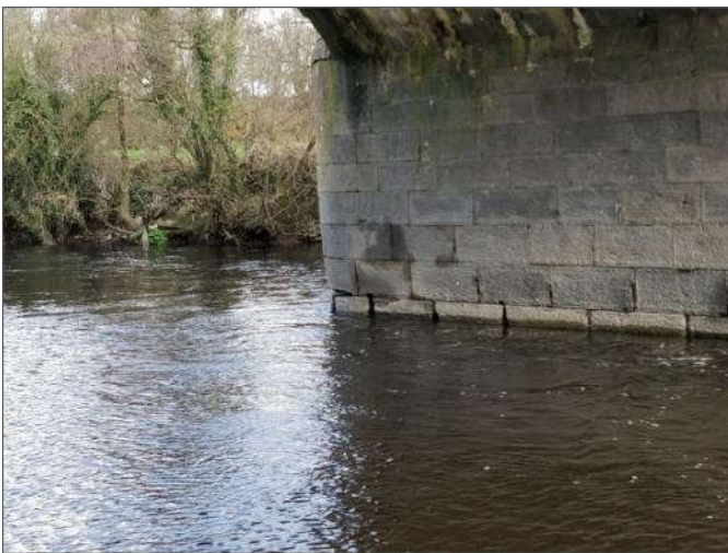
Plate 1.6 Masonry damage of north cutwater of east pier.
