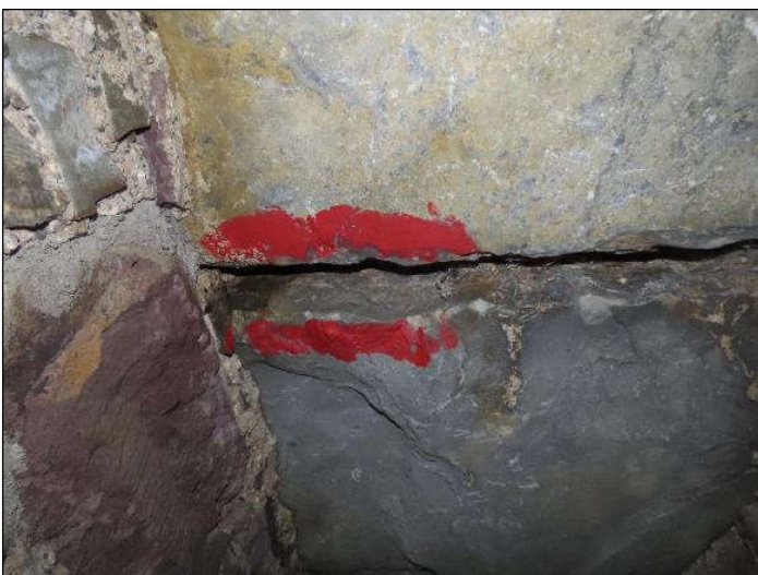
Plate 4.29 Gap between capping stones of centre span marked previously for retention for bats.
