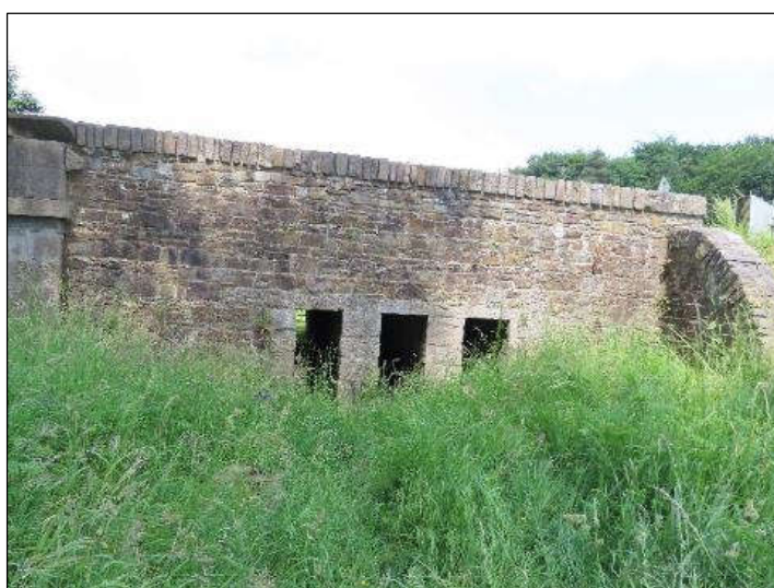
Plate 4.1 Downstream (southern) elevation of Eastern Flood Pass. The wall of Leader’s Bridge is visible on the left-hand side of the photo.
