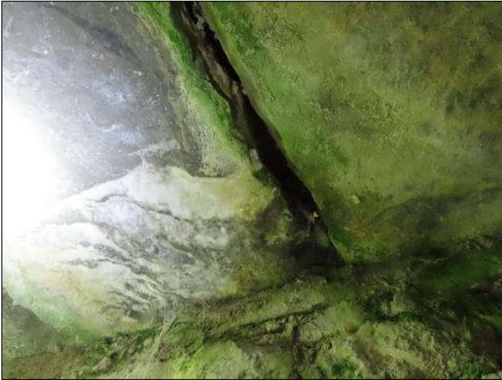
Plate 4.5 Ideal crevices for bats between capping stones of clappers – these gaps are not to be pointed.
