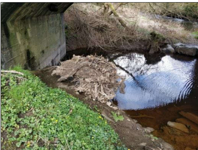
Plate 1.3 Blocked western span of Leader's Bridge.
