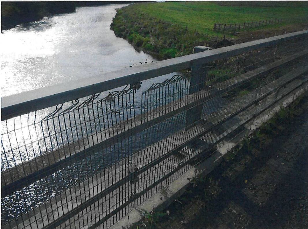
Plate 3. Damaged mesh on parapet
