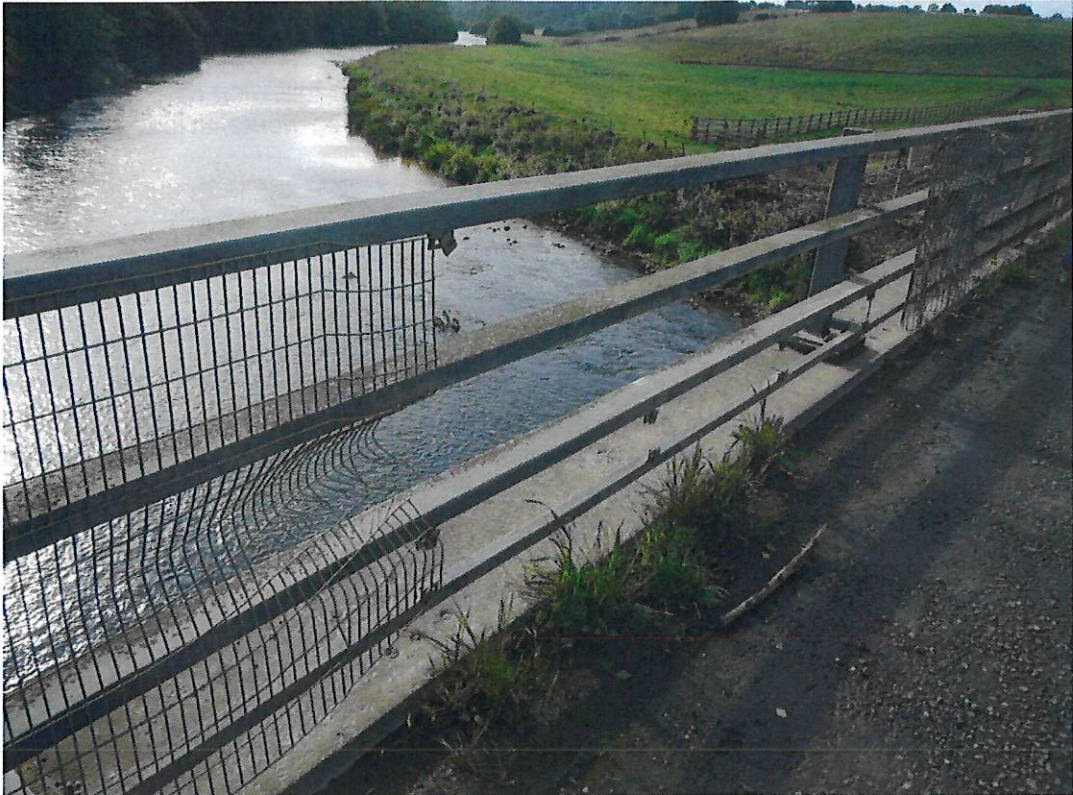
Plate 2. Damaged mesh on parapet
