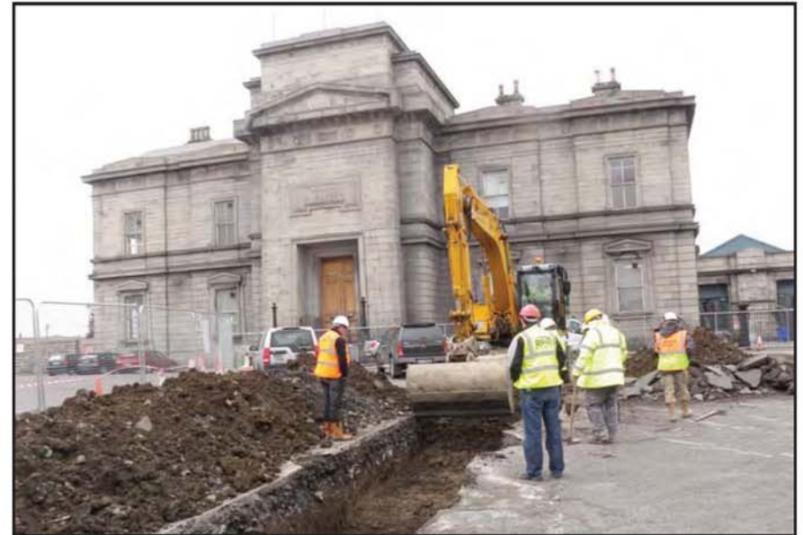
Plate 8 - Mid-excavation of Trench 2 looking towards the former Broadstone station terminal building in the background, northwest facing
