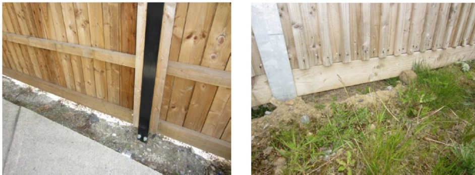
Figure B.12 - Noise Barriers with gaps underneath
