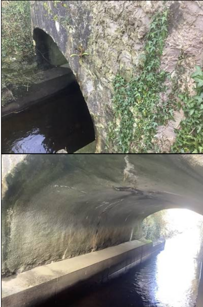
Plate 1 – Single arch masonry bridge (taken during Year 3 surveys). Plate 2 – underside of bridge.
