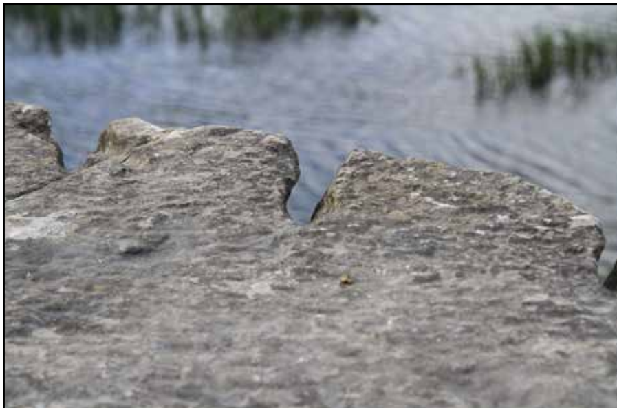
Grooves cut in parapet by ropes used to manoeuvre canal barges.
